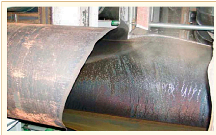
Figure 2-4: Main Feedwater Piping Rupture at Mihama 3, in August 2004 [Kepco, 2005].
